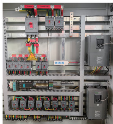
总控制电柜 Main control cabinet
